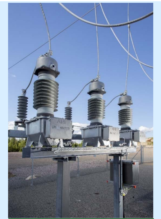
Plate 5.16 - Typical Voltage Transformer Image: ©ABB
