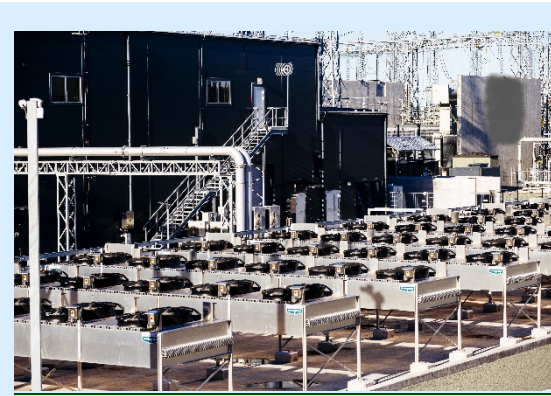
Plate 5.23 – Typical Outdoor Heat exchangers Image: ©GE
