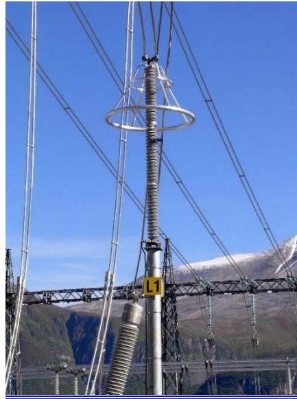
Plate 5.7 – Typical HV Surge Arresters Image: ©ABB
