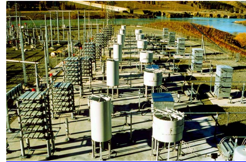
Plate 5.11 – Typical AC Switchyard Harmonic Filters Image: ©ABB
