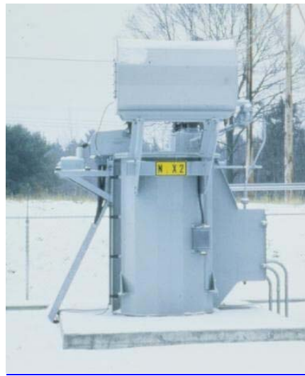
Plate 5.12 – Typical Auxiliary Power System Image: ©ABB
