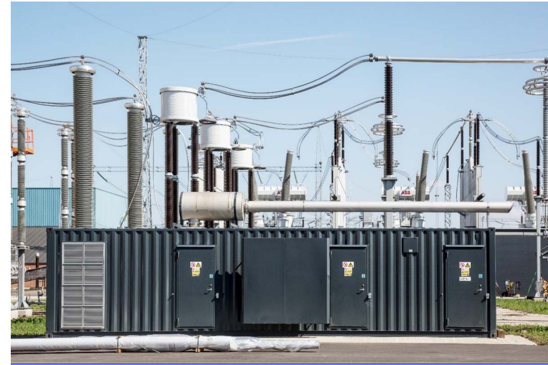
Plate 5.13 – Typical Diesel Generator Image: ©ABB
