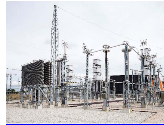
Plate 5.8 – Typical Lightning Masts Image: ©GE
