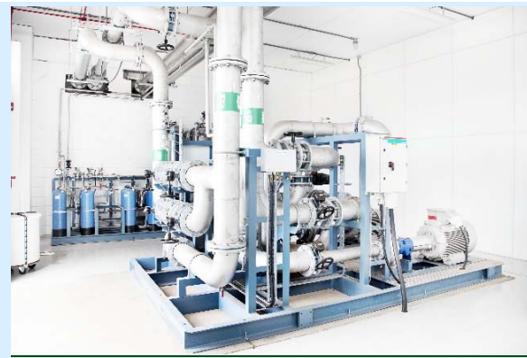
Plate 5.22 – Typical Water Pumping Station Image: ©ABB
