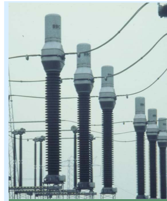
Plate 5.15 – Typical Current Transformer Image: ©ABB
