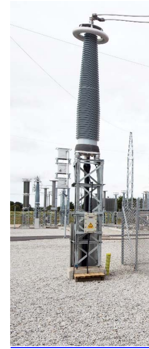
Plate 5.6 – Typical 400kV Cable Terminations Image: ©GE
